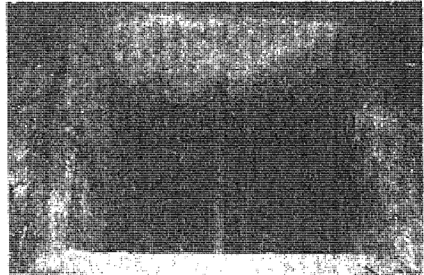
Fig.2a. Injection well at site-2
